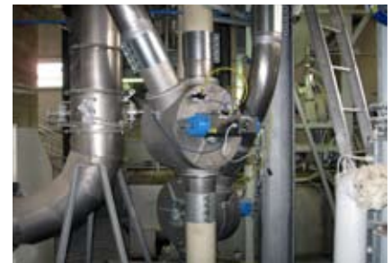
Drum-type diverter valve in pneumatic conveying system
