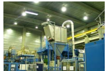
Dust collector in car tank factory
