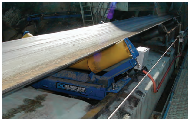
Single Idler B150 Belt Weigher on aggregate conveyor
