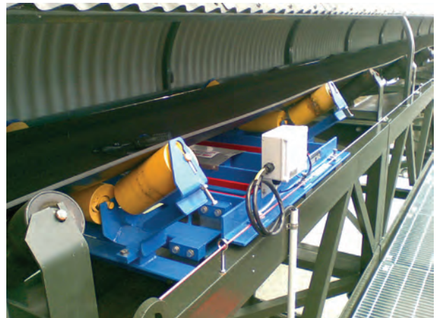
New B152 installation on coal conveyor
