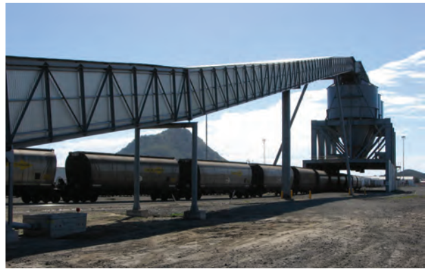
Enclosed installation on train loading coal conveyor
