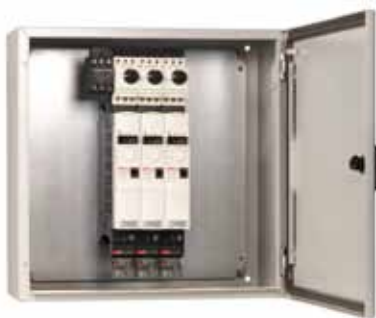
Power supply and protection for several drives by means of a busbar and circuitbreakers.
