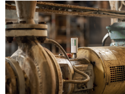
Paper mill: OPTIME CM does well in motor monitoring
