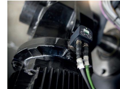
Logistics center: SmartCheck monitors rack feeder motors
