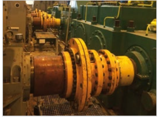
Shear pin gear couplings in steel mill
