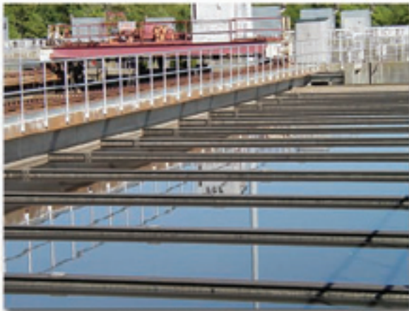
Closer view - 36 ft wide Clarifier with SAV 709 Chain
